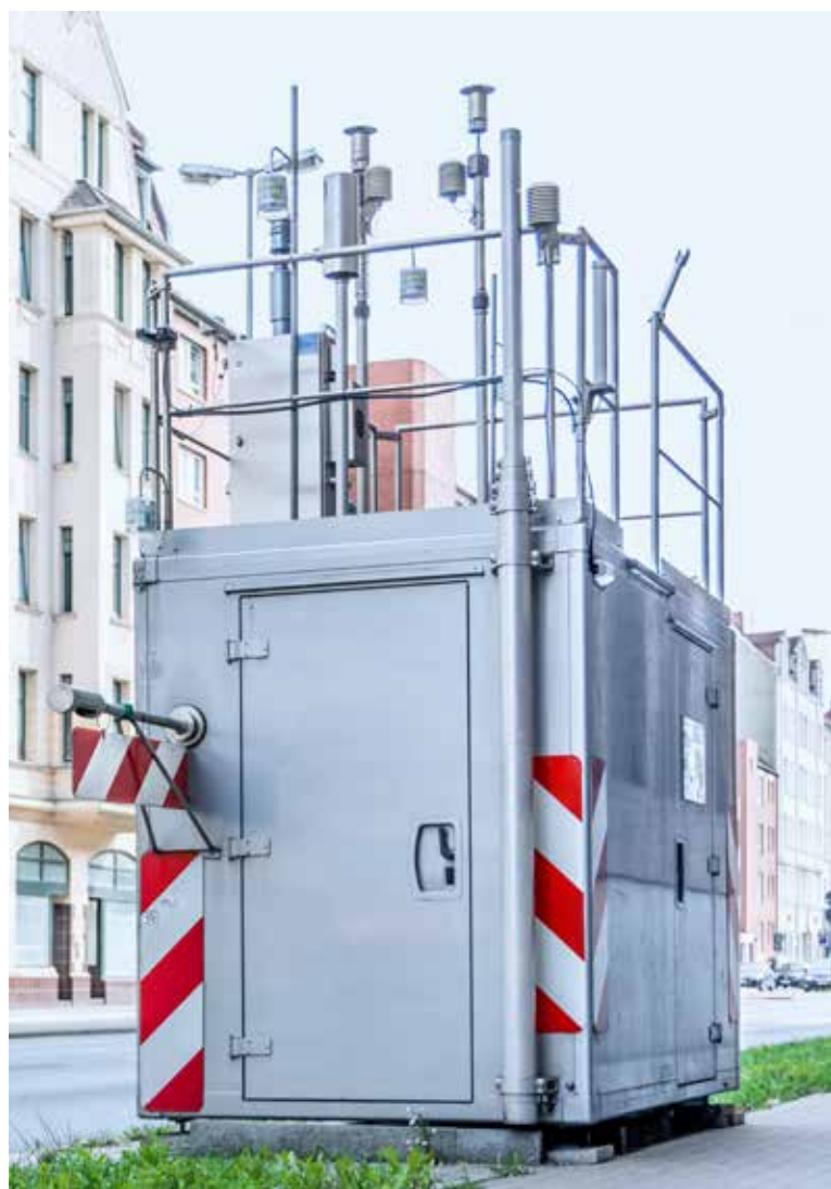
Measuring station for immission monitoring
